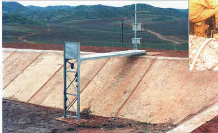
Balancing dam at Pongola with telemetry and low level switches.
