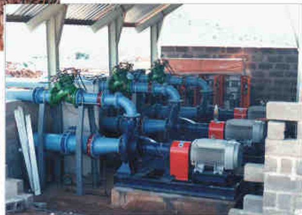
225 kw Pump station at Pongola. Fully automatic with telemetry, pump control valves, surge valves and low water protection.
