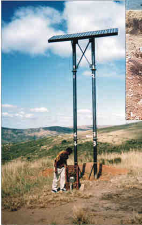
Solar panel powered pump for rural domestic water supply in the Zululand District Municipality area.
