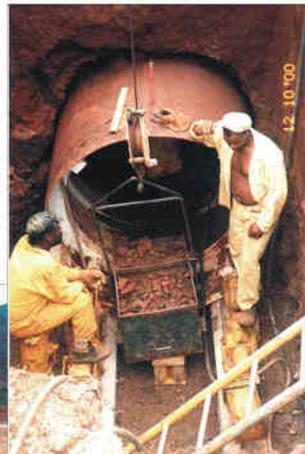
Pipe jacking of 1,4m diameter concrete pipe sleeve under the N2 road, Mkuze.
